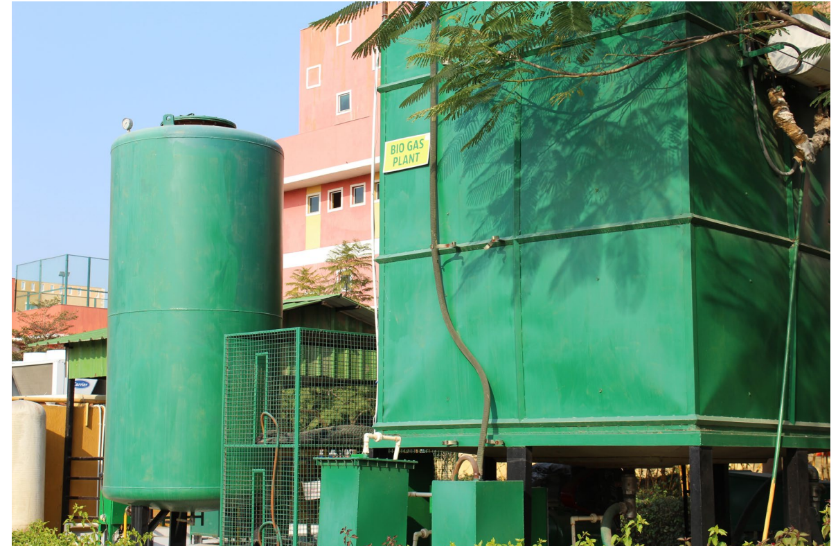
Bio-Gas generation system 30kg of Gas per day with 500 kg of Kitchen waste
